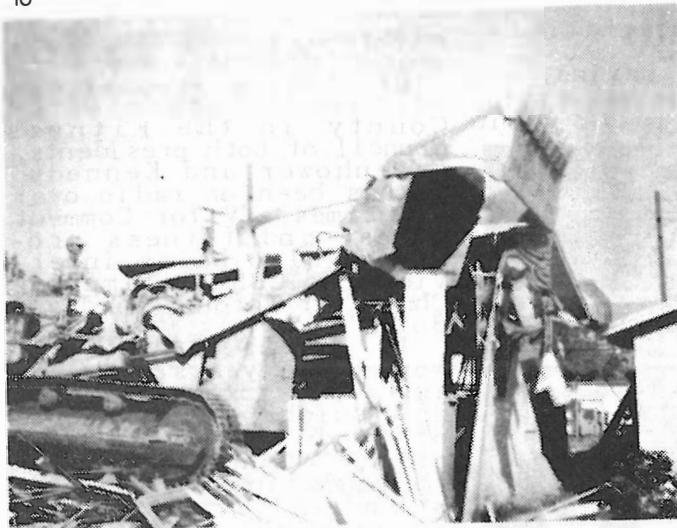
HUGE CAT JAWS DROP ON HOUSE, GRIND IT TO KINDLING. THEN GIANT RAKE PULLS DEBRIS OUT. LOADS IT ONTO BIG WAGON BOUND FOR DUMP.
